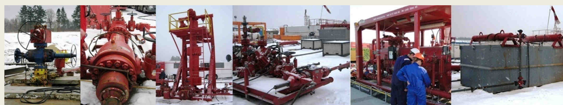
WELL HEAD COARSE SEPARATOR SAND CATCHER MANIFOLD SEPARATOR TANK
